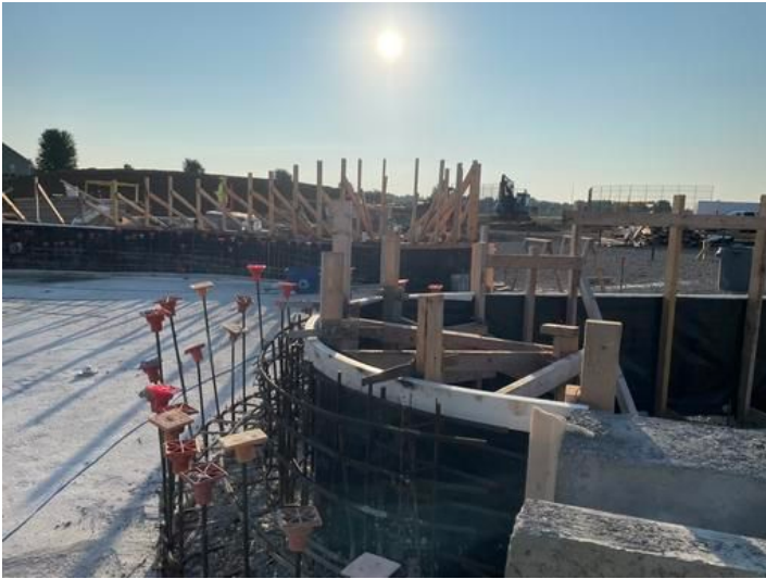
Installation of Walls on the Lazy River Taken on Jul 6, 2023, 7:00 AM CDT Added on Jul 6, 2023, 7:49 AM CDT Added by andrew gordon
