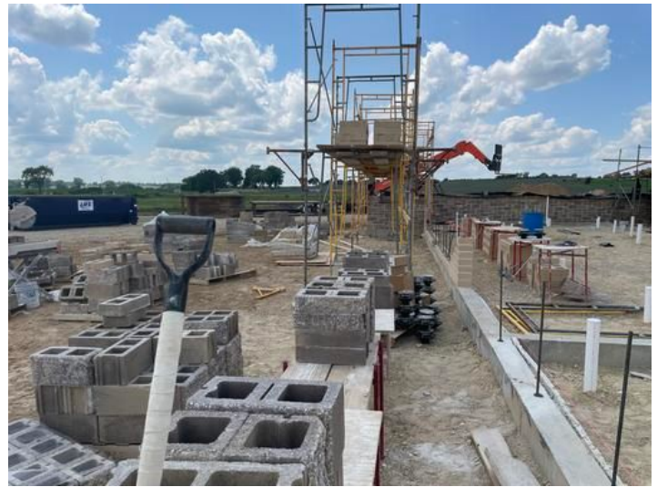
Preparing for Exterior CMU installation on the south side Bath House. Taken on Jul 6, 2023, 2:06 PM CDT Added on Jul 6, 2023, 2:26 PM CDT Added by andrew gordon
