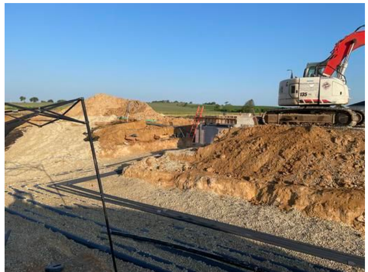
Installation of underground pool pipes to Equipment/ Pump House Taken on Jul 6, 2023, 7:02 AM CDT Added on Jul 6, 2023, 7:49 AM CDT Added by andrew gordon
