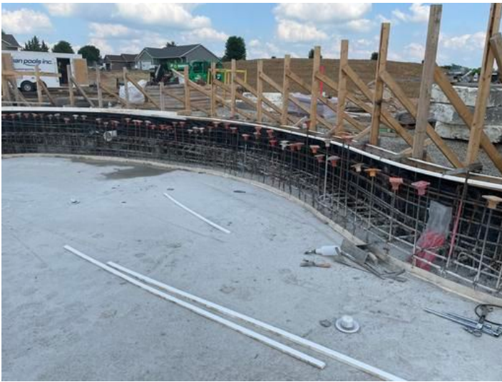
Installation of Lazy River wall rebar Taken on Jul 6, 2023, 2:07 PM CDT Added on Jul 6, 2023, 2:26 PM CDT Added by andrew gordon
