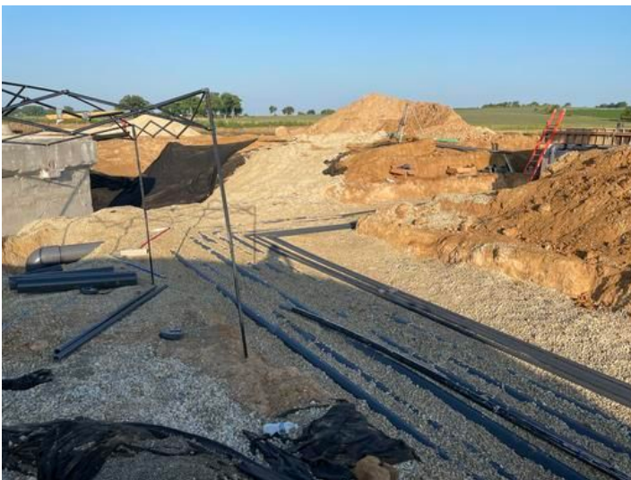
Installation of underground pool pipes to Equipment/ Pump House Taken on Jul 6, 2023, 7:02 AM CDT Added on Jul 6, 2023, 7:50 AM CDT Added by andrew gordon
